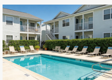
Swimming Pool Water Treatment
